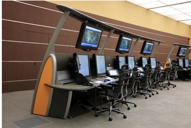
Air Traffic Management System
